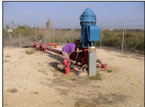
FIGURE 2.4: Water level measurement in a production well.
