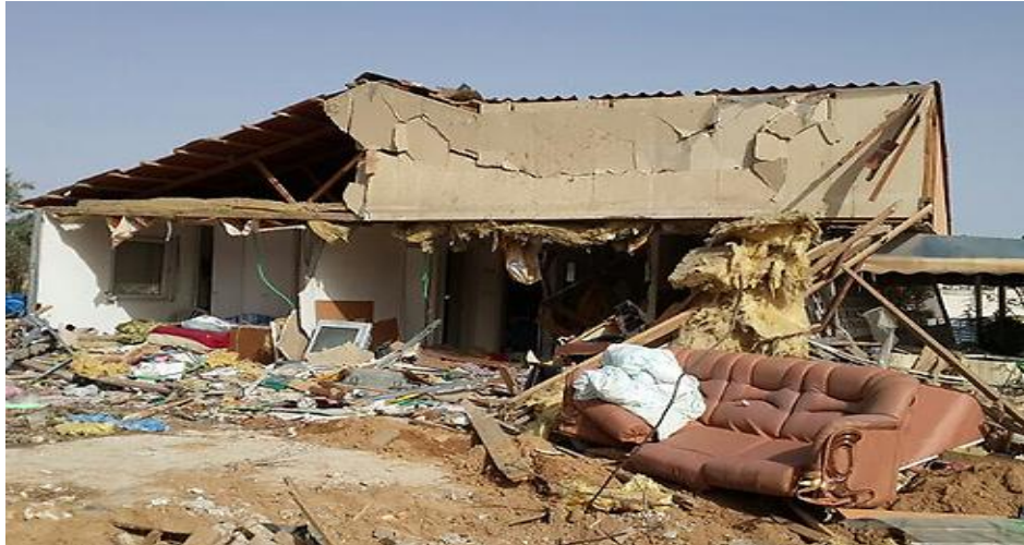
Above: A house in Be’er-Sheva after a direct hit from a rocket from the Gaza Strip on July 12, 2014. (Source: IDF)
