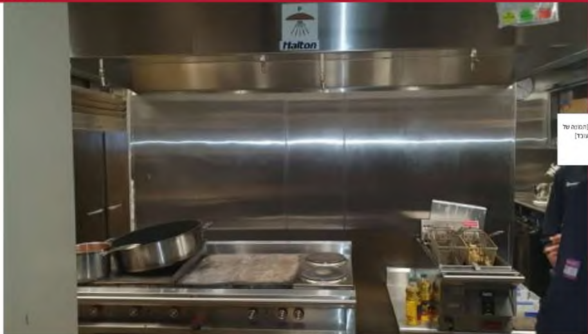
Figure 1: Metal pot following the grease fire.
