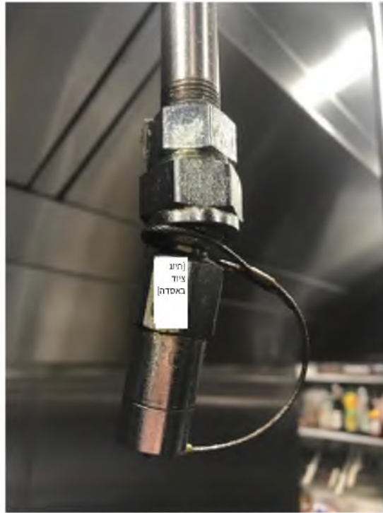
Figure 2 (above) shows overhead fire suppression system.
