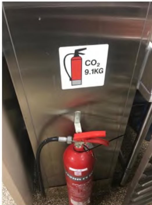
Figure 3 (above) shows the CO2 extinguisher next to the stove.
