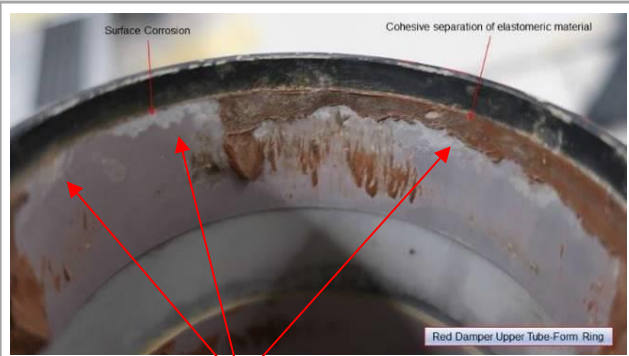
Figure 3 - Red damper tube form housing interior.
