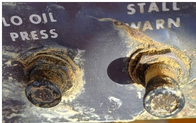
Figure 8 - Stall Warning System circuit breaker
