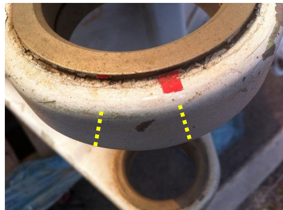
Example of Bushing Movement
